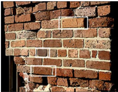
top: Installation of brick patching material (not finished yet). Three different colors of mortar were used. bottom: Next day close-up. The brick repairs are very hard to find.
